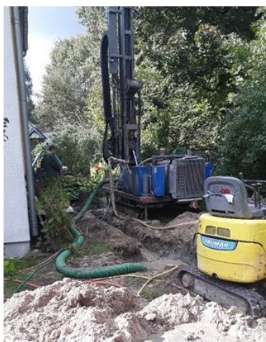
Ground heat exchangers
