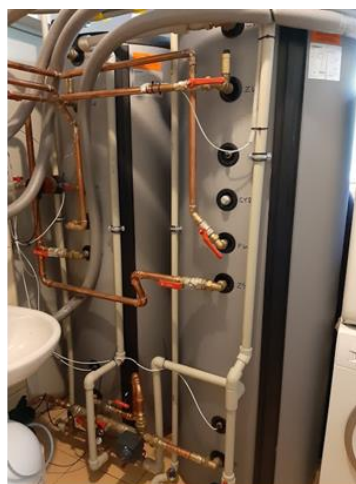
Buffers in boiler room
